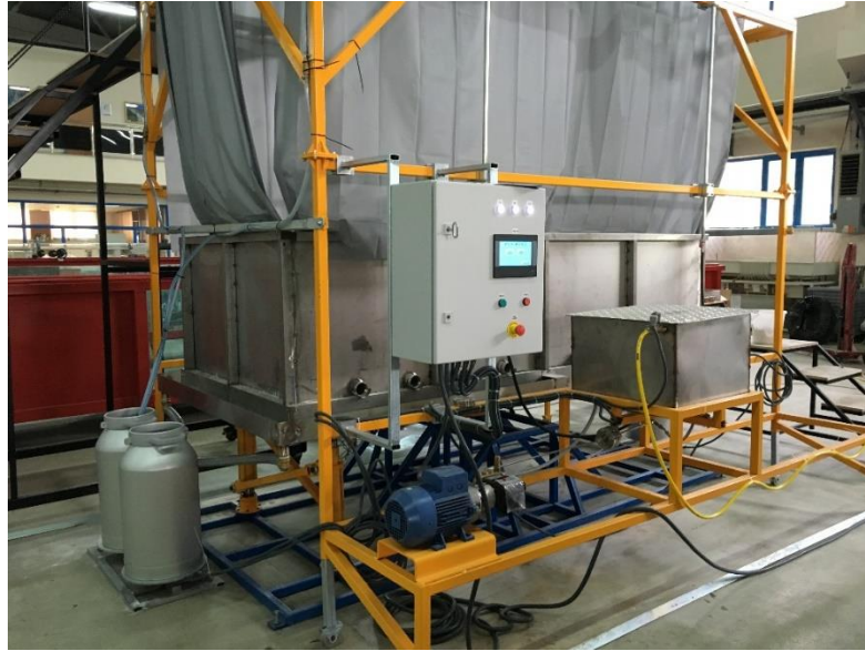
Figure 5.4 Details of PLC Control Panel, Motor, Pump, and Orifice Meter
