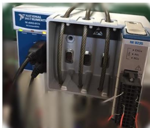
Figure 3.8 Data Logger and its chassis
