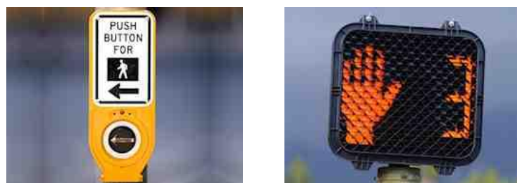
Figure 3.27 Accessible Pedestrian Signals [66].
