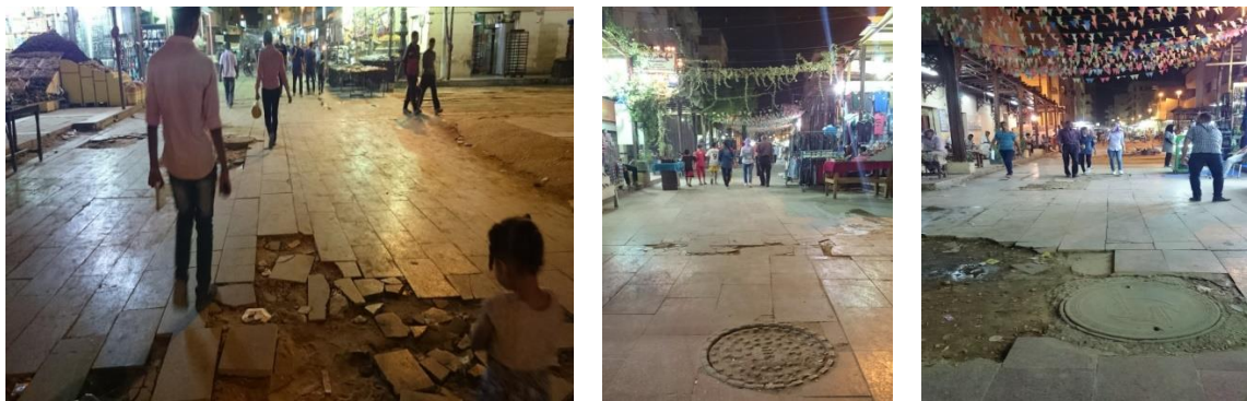
Figure 4.35 The street's floors are uncomfortable, unstable and slipping in some of its sectors.
