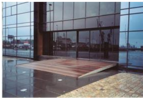
Figure 3.32 This entrance is virtually impossible to distinguish from adjacent window panels [62].
